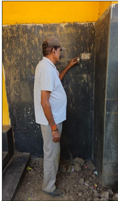
Activation of electrical fire siren
